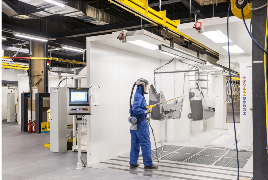
The recoating stations with floor aspiration are spacious, light and offer quick access to the controls.
