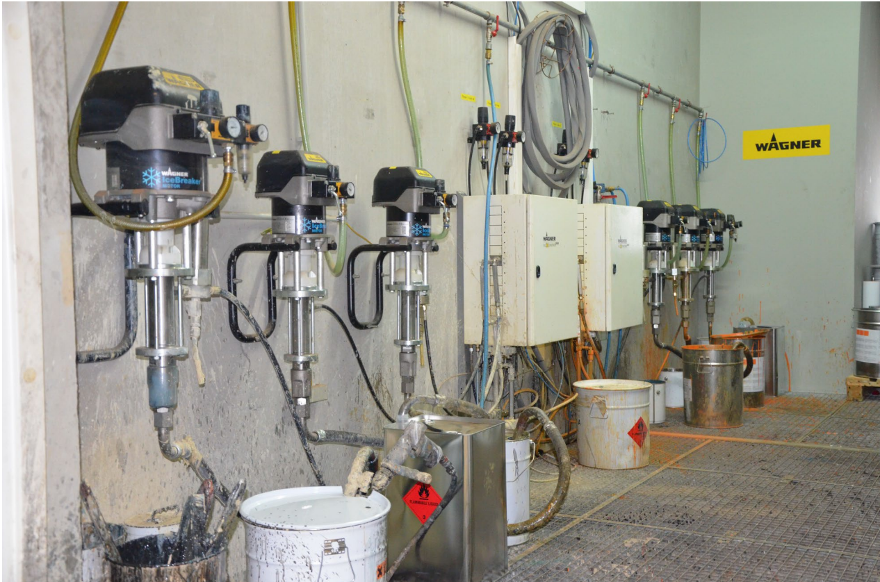
The paint shops at Springer are supplied by several pumps and mixing and dosing systems.
