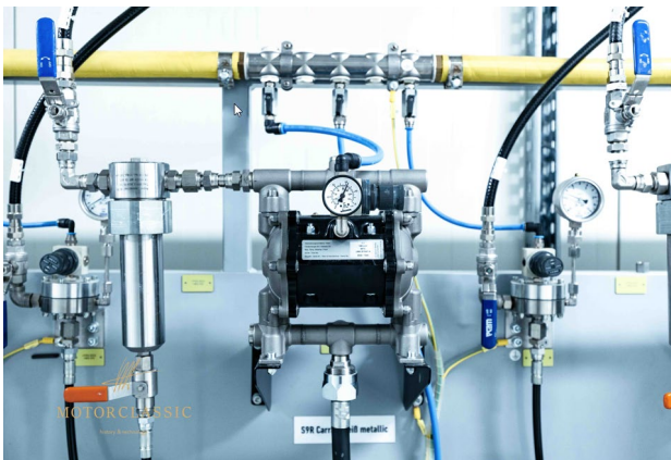
Paint supply with ZIP 52 double diaphragm pumps and various drum lid lifting stations
