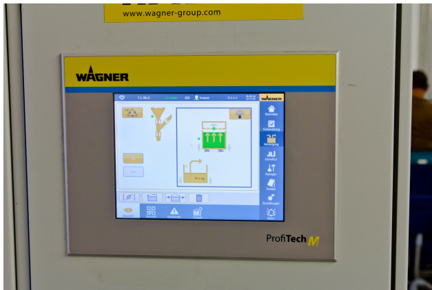
Photo: User-friendly touch-screen menus support the powder coating system's efficient operation
