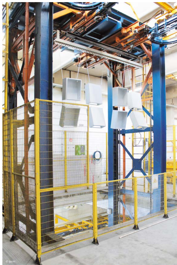
The lowerator is coupled with the workpiece-carrying load bars and takes them to the ground floor.
