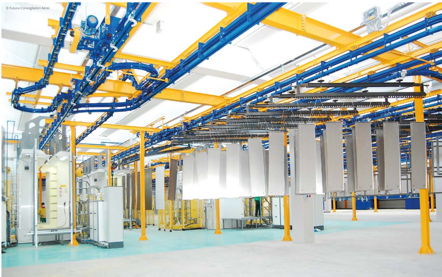
The power & free conveyor and the 3 Wagner booths.
