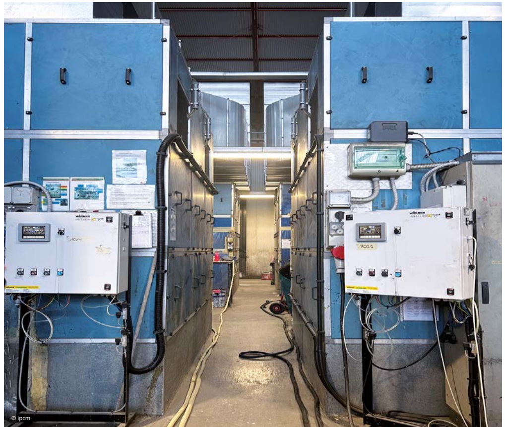
The 2 Wagner Intellimix units for paint mixing and dosing.
