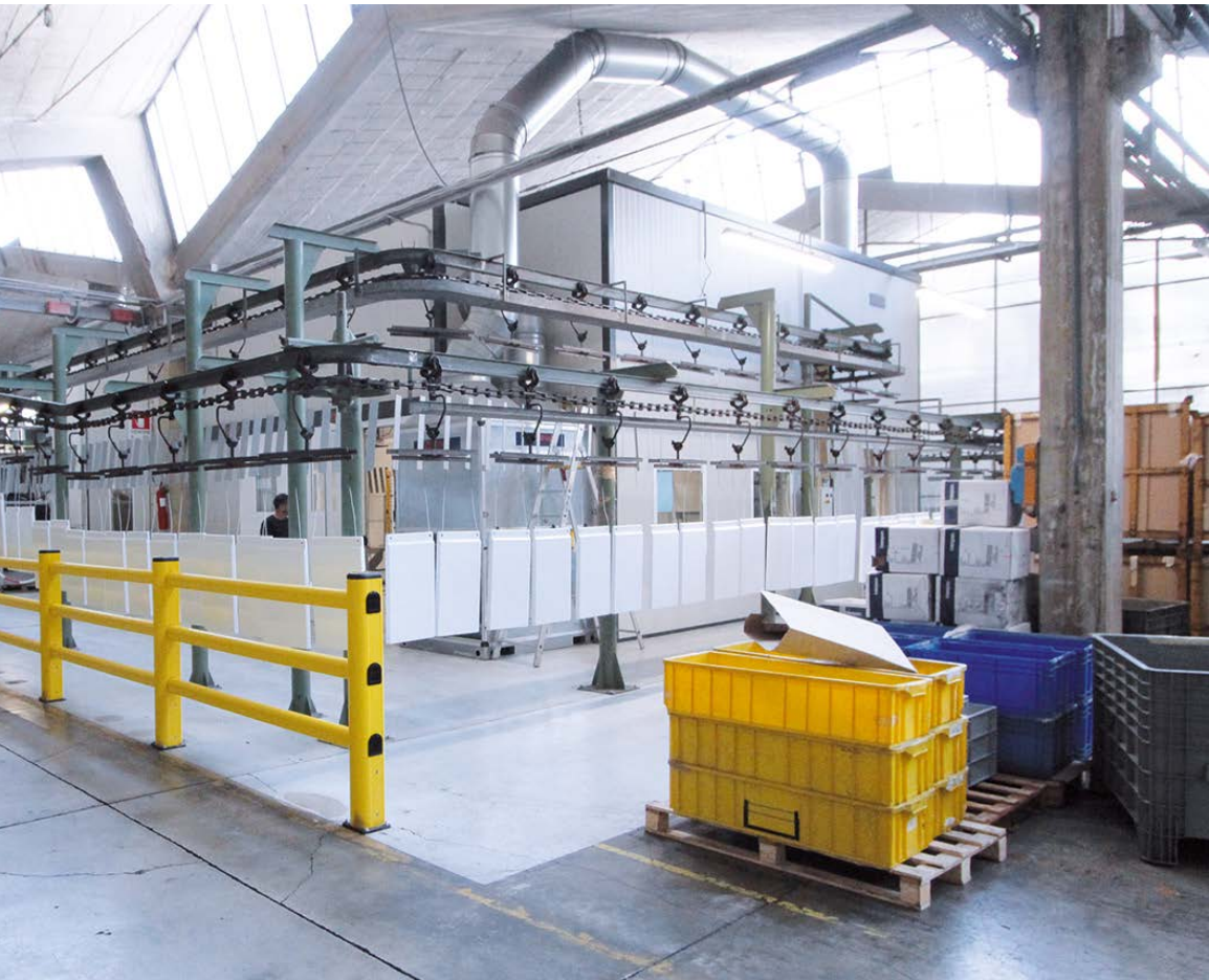
Top left: oven cavities entering the pre-treatment tunnel.
