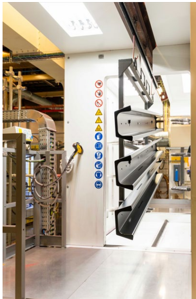
Powder coating system at VBG Truck Equipment (image source: Ytforum)
