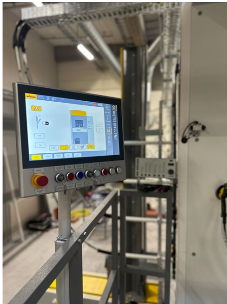
WICOS control system for the monitoring of the coating process
