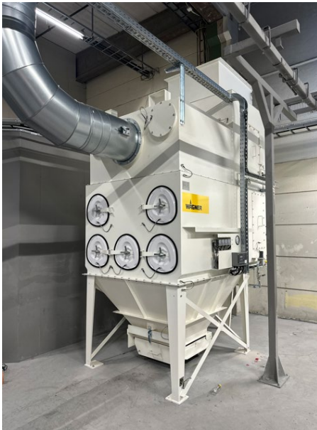
Final filter of the new powder coating line
