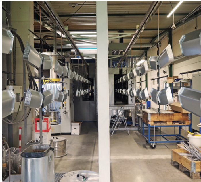
The system is installed in a very confined space.
