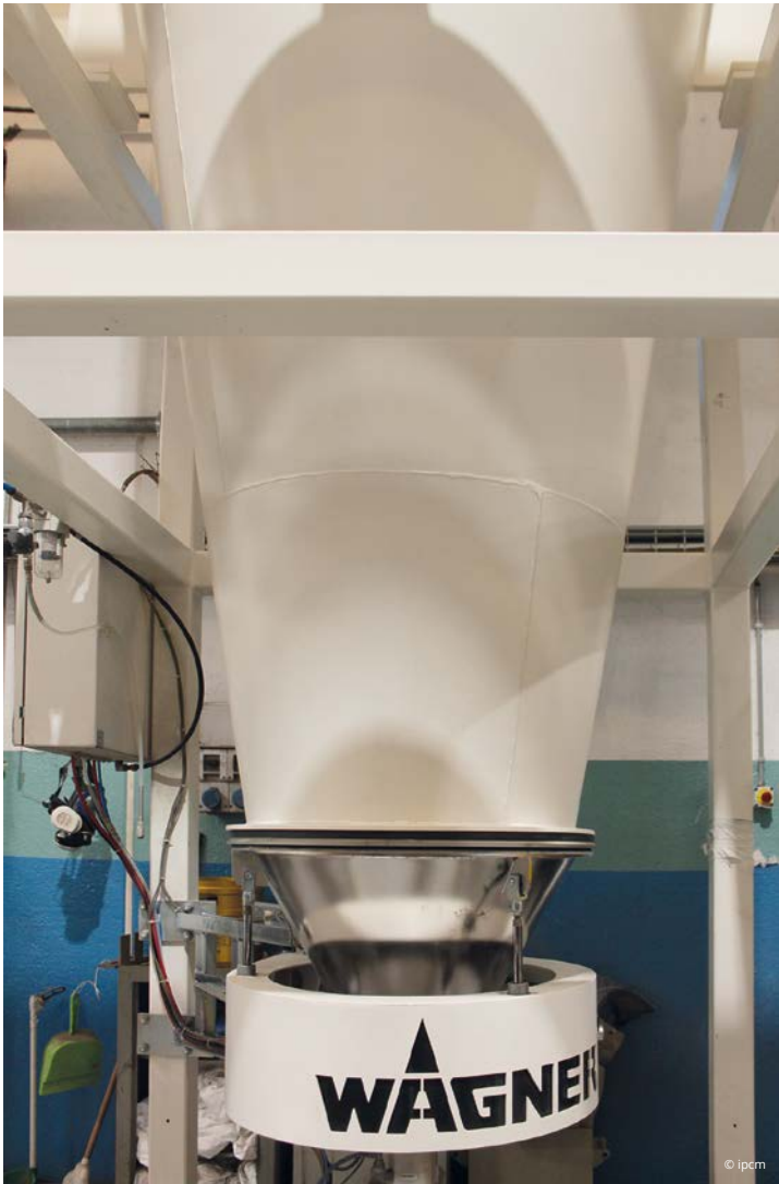
The cyclone for powder recovery.
