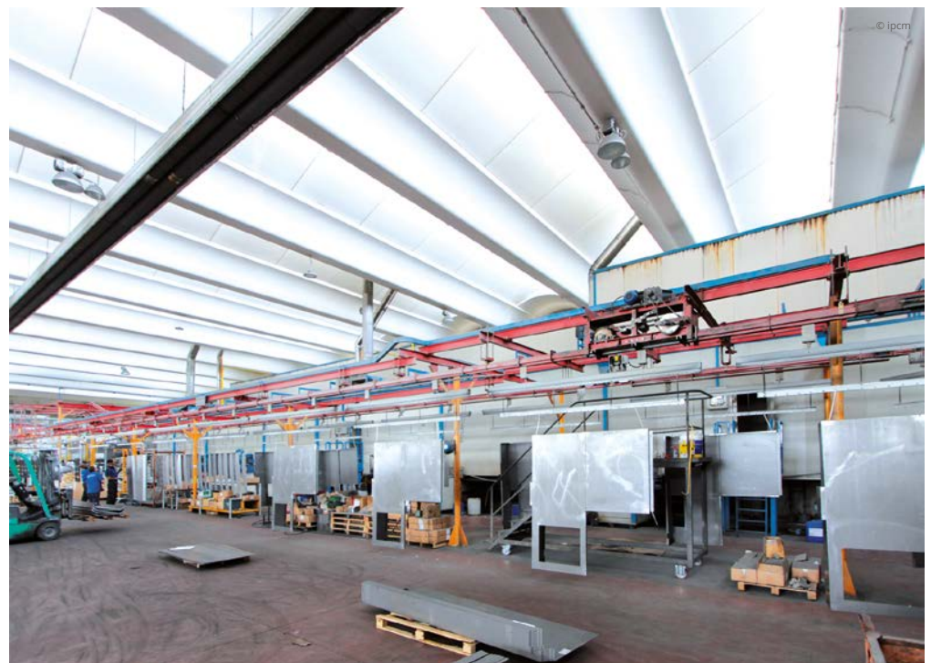
General view of the coating line designed by Imel and built by Nord Laser itself.
