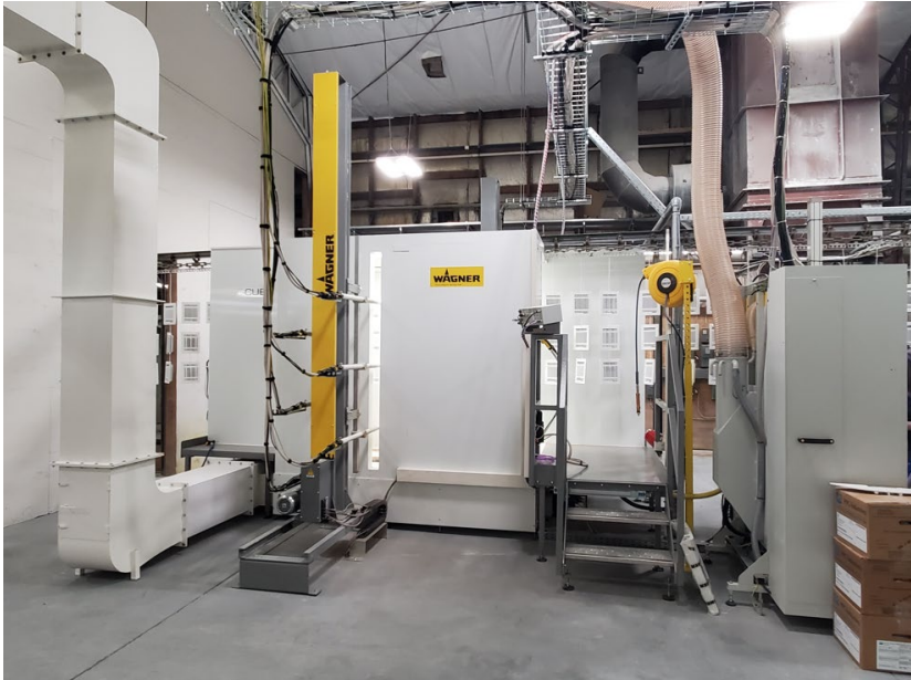
New E-Line system at Shoemaker with booth, powder center, cyclone and filter
